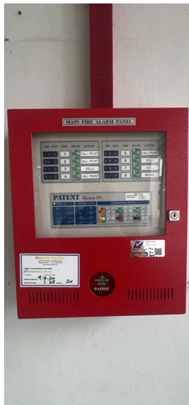
A well maintained Patent System 88i fire alarm panel c/w valid servicing sticker and no faults on panel. Photo credit: Fiready Pte Ltd
