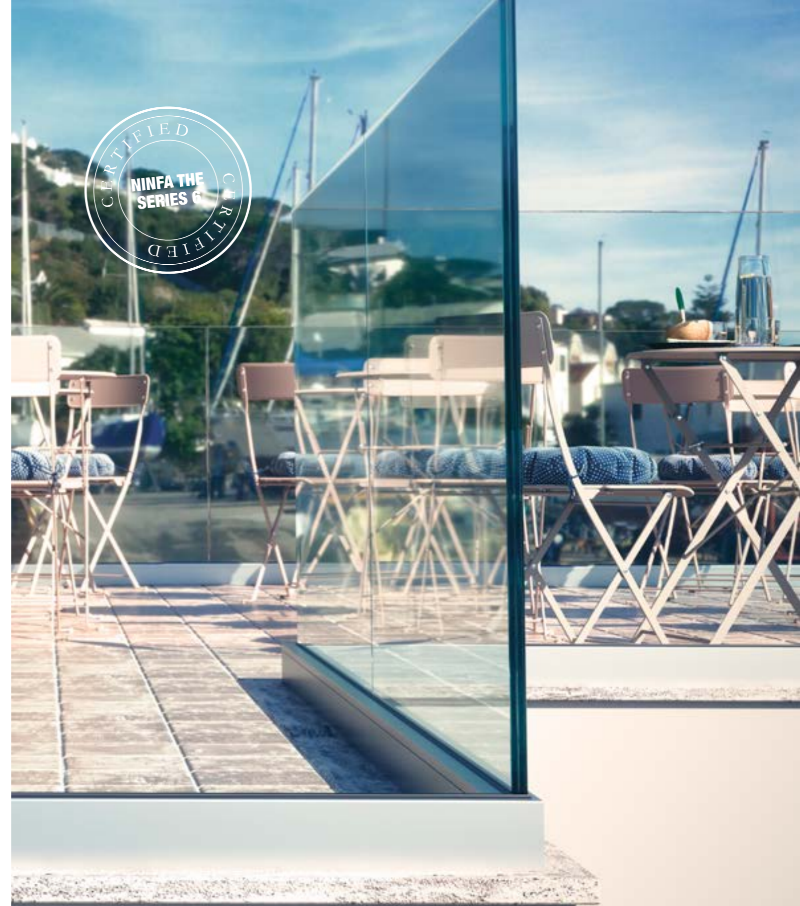
Example of NINFA 56 with 8+8 H. 100 glass positioned in an environment with a "fall into the void" of less than 80 cm.
